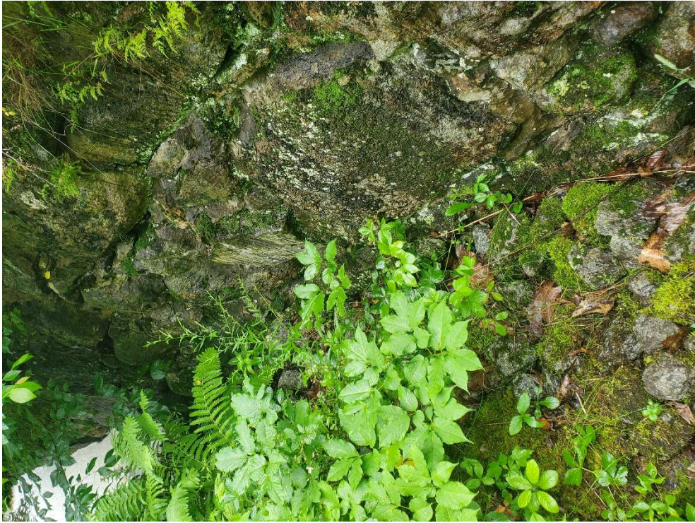
Photo 11 – No seepage observed on downstream toe of Ashuelot Pond Dam during high water event July 10, 2023
