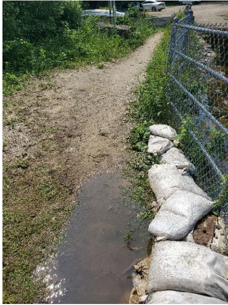
Photo 13 – Sandbags placed by M&K to prevent overtopping of dam in low area to the right of the gatehouse
