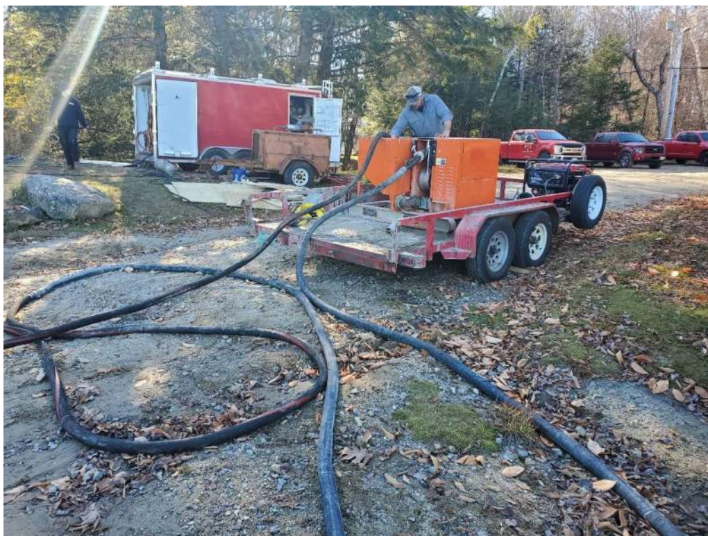
Photo 2 – M&K setting up the peristaltic grout pump November 3, dive crew control trailer in background
