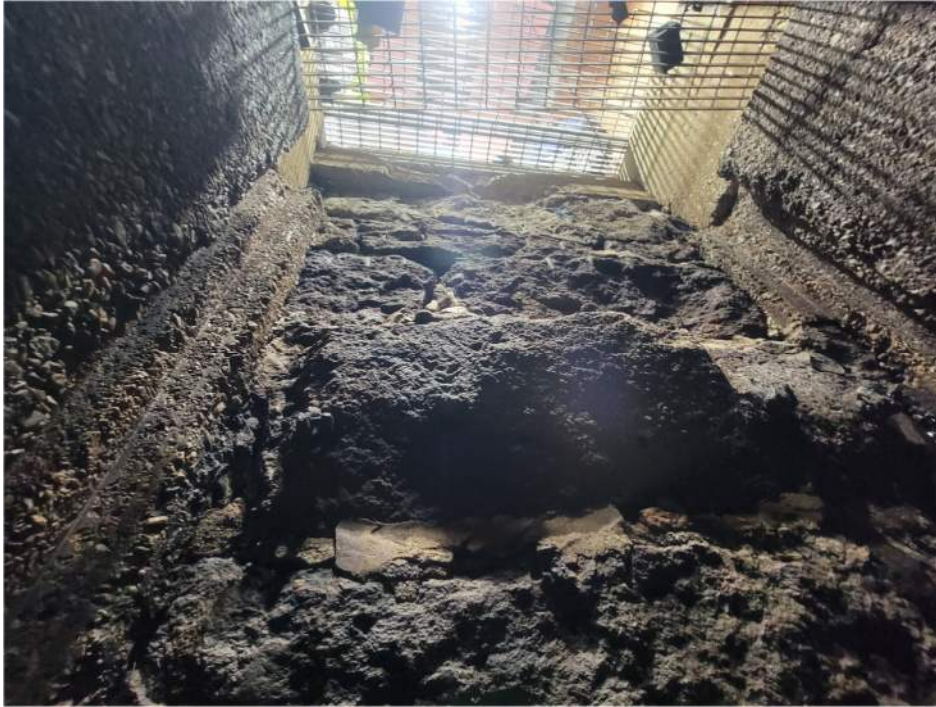
Photo 3 – Ashuelot Pond Dam Gate House – interior face of downstream gate house water pit (elevation view of Wall D facing downstream)
