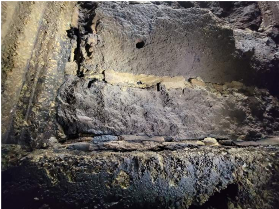
Photo 4 – Ashuelot Pond Dam Gate House – interior face of downstream gate house water pit above outlet (elevation view of upstream face of Wall D facing downstream)
