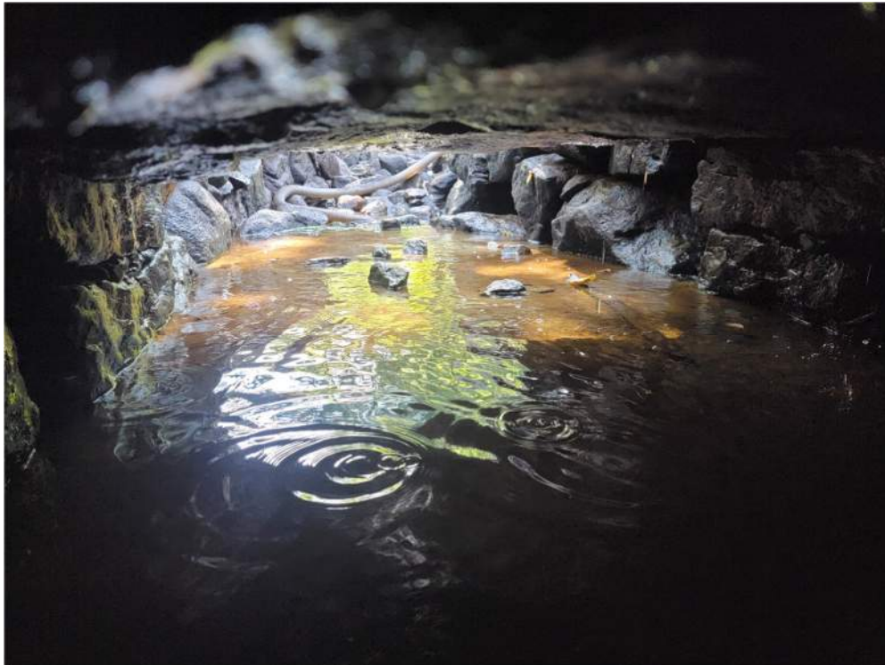
Photo 8 – Ashuelot Pond Dam Gate House – outlet channel of gate house (base of wall D)
