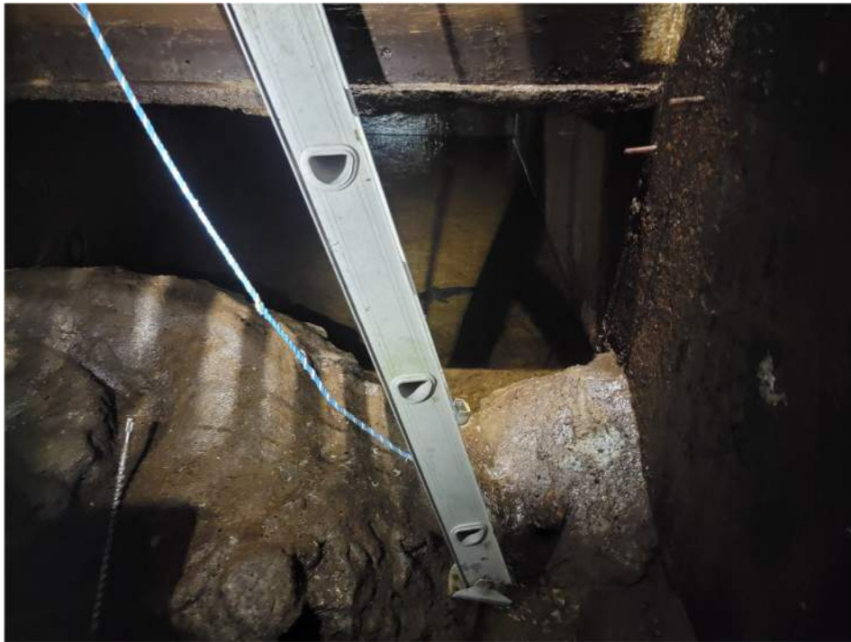
Photo 6 – Ashuelot Pond Dam Gate House – concrete over-pour at downstream end of gate house inlet (to be removed) (Base of Wall A)
