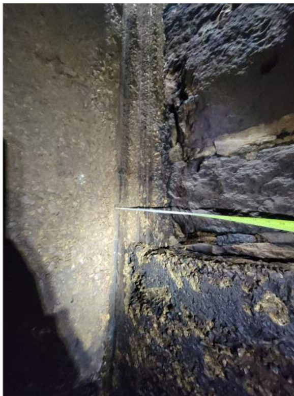
Photo 2 – Ashuelot Pond Dam Gate House – downstream left corner at former stoplog bay (elevation view facing downstream at corner of walls C & D)
