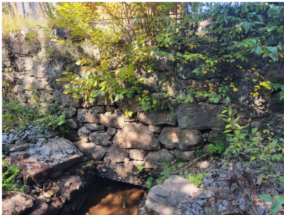
Photo 9 – Ashuelot Pond Dam Gate House – downstream exterior face of gate house and dam at outlet
