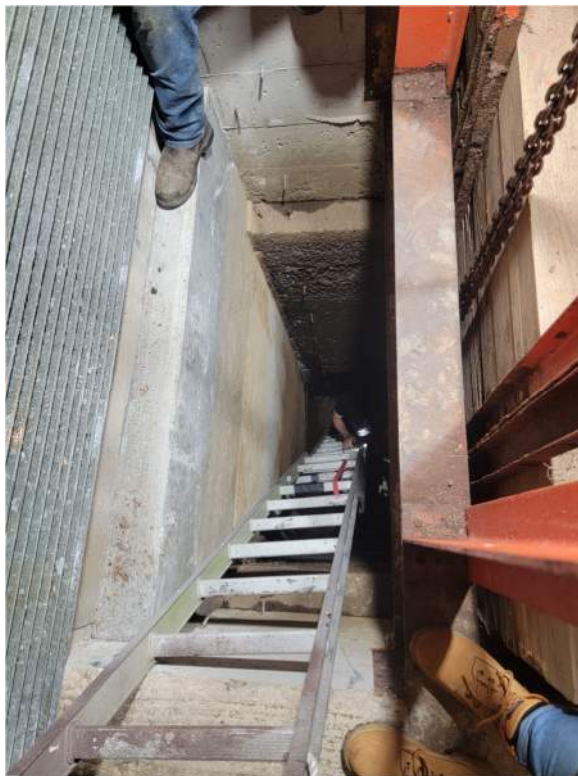
Photo 1 – Ashuelot Pond Dam Gate House – interior face of upstream gate house water pit (Wall A from Figure 1)
